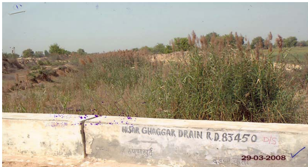
Non-functional Hisar Ghaggar drain at RD 83450
